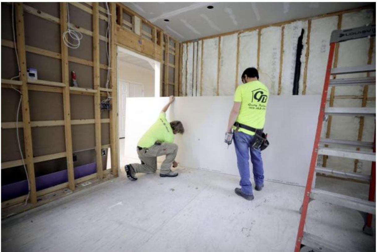
Chris Keener, left, and Bill Poette, both carpenters with Geary Builders, install drywall at a job site in Lenox. The company has seen increasing wait times, both in the lead up to projects and to complete them, because of a lack of skilled laborers in Berkshire County.
